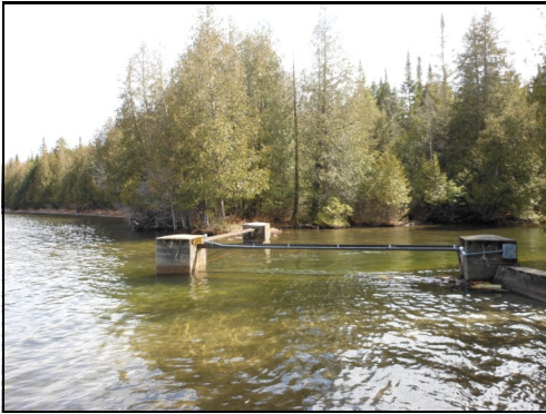
The outlet at the south end of Seymour taken from the location of the pins on April 12, 2012 when the lake level was 13 inches above the low pin. The outlet structure has 3 concrete stanchions connected by dual railroad irons. Originally these irons supported fish screens which were later removed.
